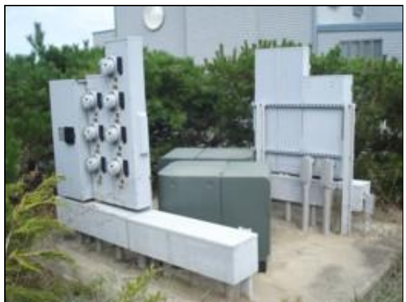
Photo #6. Electrical System
