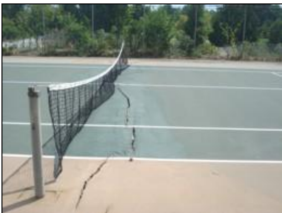
Photo #5. Tennis Court - Cracks
